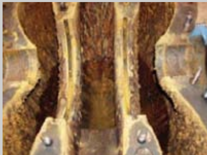
Corroded Pump Volute
