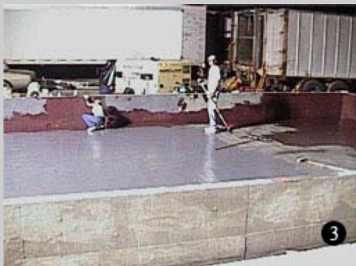
Belzona® 4311 coat interrupted.
